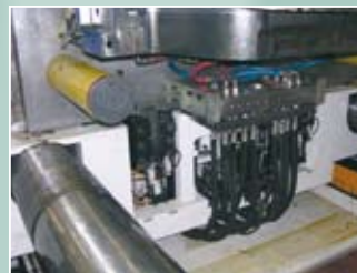
Horizontally mounted multi coupler to connect all utility connections from below.
