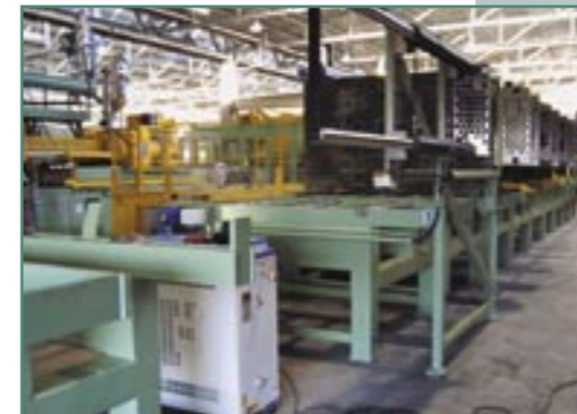
The storage systems also include a preheating station, which is shown here during the installation period.
